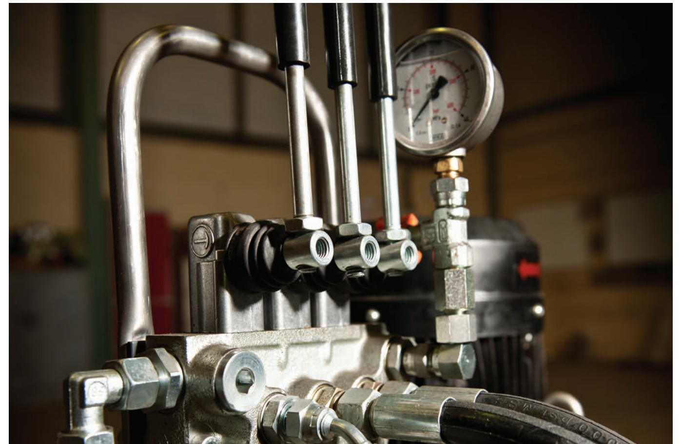
Hydraulic Curtain Adjustment and Frame Opening
